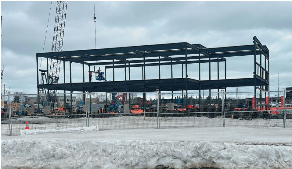
The Ontario Power Generation ( OPG ) new building facility at the Innova Business Park
